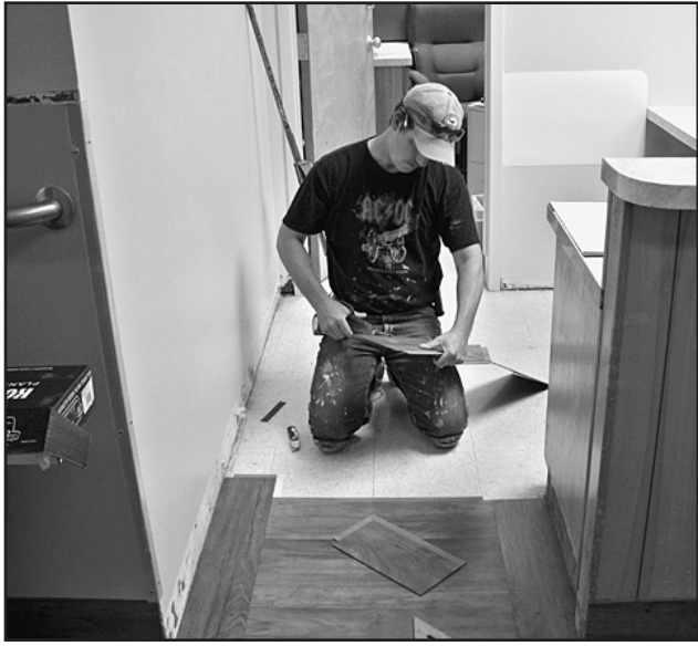
NEW FLOORS —Richard Powell of Rp Construction lays new flooring with a hard wood look at Haskell Memorial Hospital.
