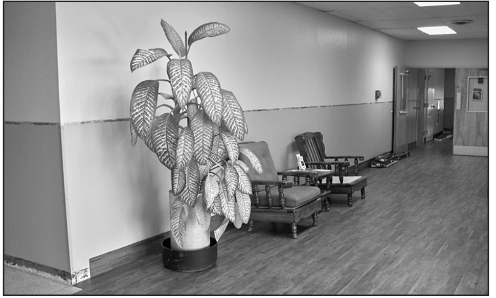
REMODEL PROJECT —A remodeling project is in progress at Haskell Memorial Hospital including new paint, flooring and trim along with new upholstery for the lobby furniture. Patient rooms are also being updated.
