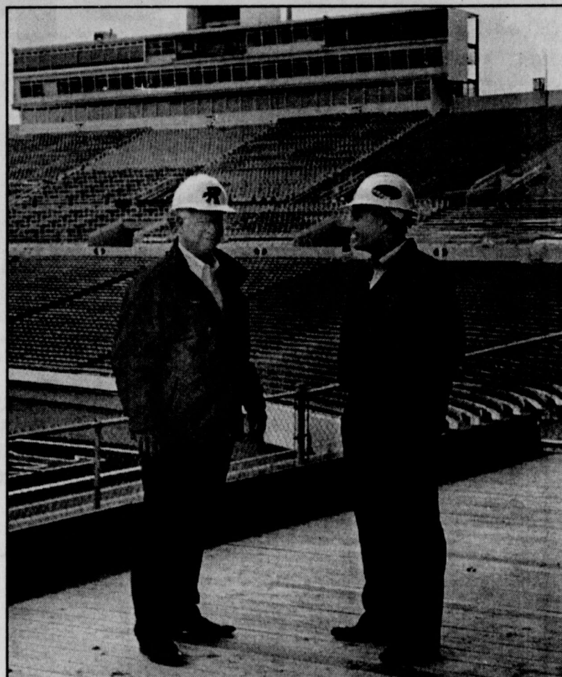
Emmett Rogers, administrator of construction for Facilities, Planning and Construction, left, and Jones SBC Stadium renovation project manager Robert Cameron, discuss the renovations in the north end of the stadium.
