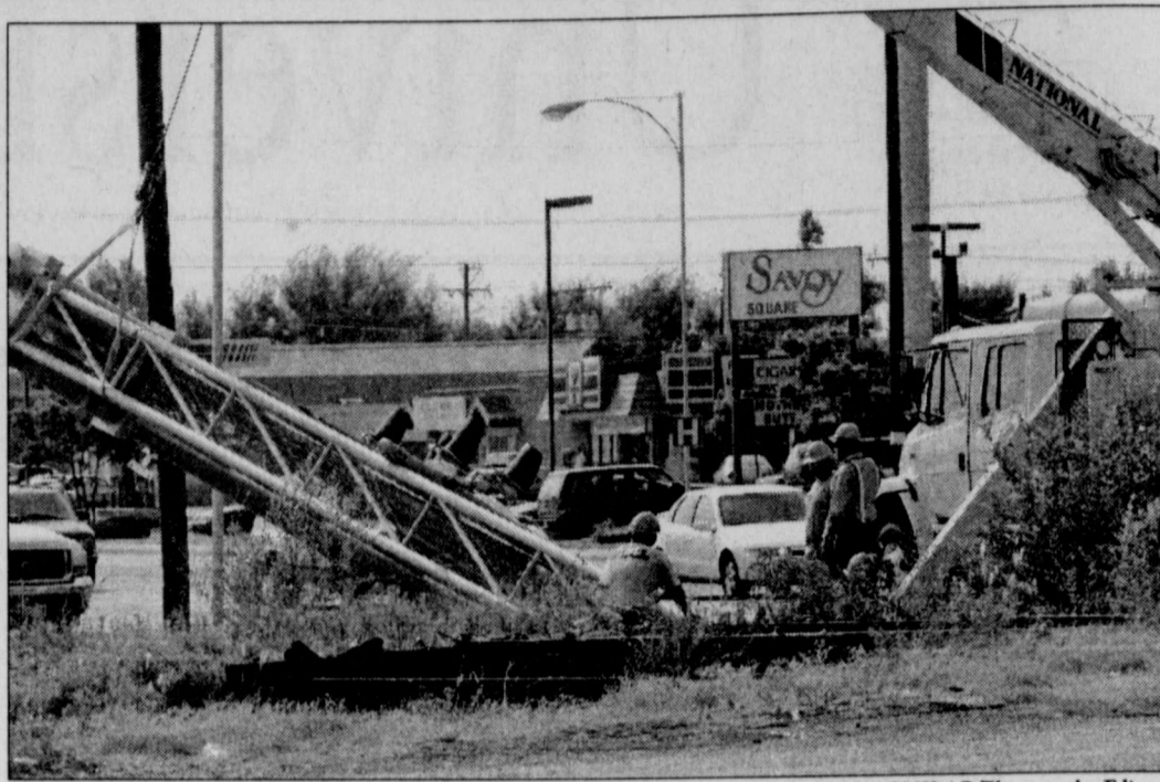
CREWS BEGIN THE removal of the crossing signals along Brownfield Highway to make room for the Marsha Sharp East/West Freeway. Workers have been removing the railroad throughout summer.
