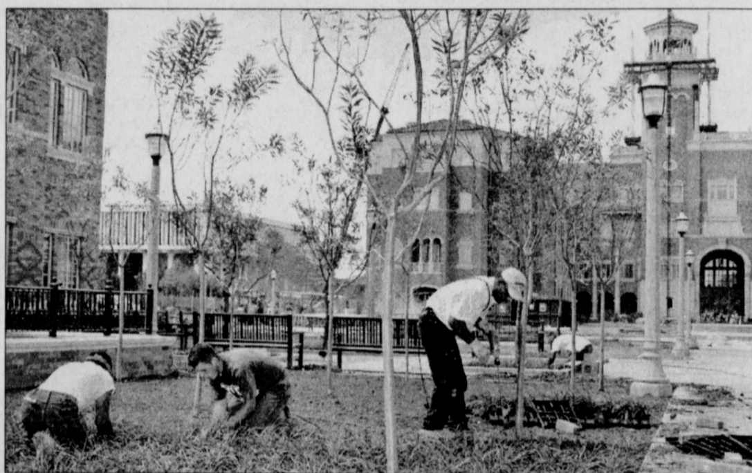
WORKERS LANDSCAPE THE courtyard between the English/Philosophy building as the construction on the complex nears completion.
