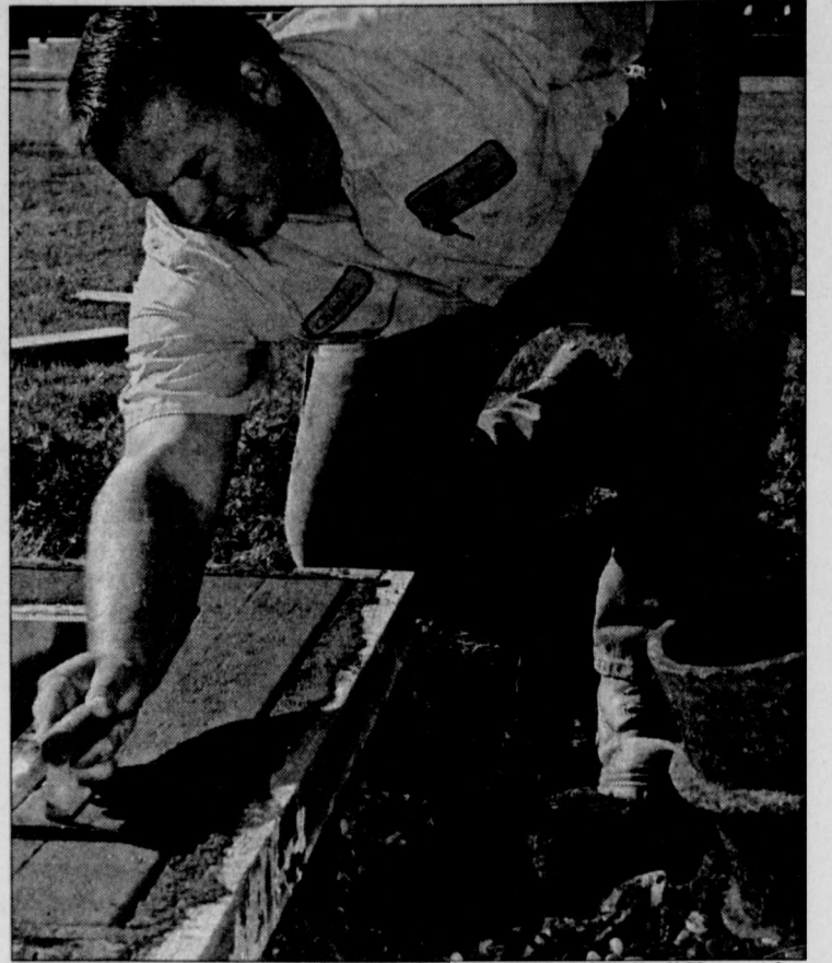
JENNA HANSEN/Staff Photographer CHARLES RIEGEL, A member of the grounds maintenance team nicknamed "Roadwarriors," smoothes concrete on an electrical base that serves as the power supply for the Christmas tree that will be placed on Memorial Circle for the holidays.
