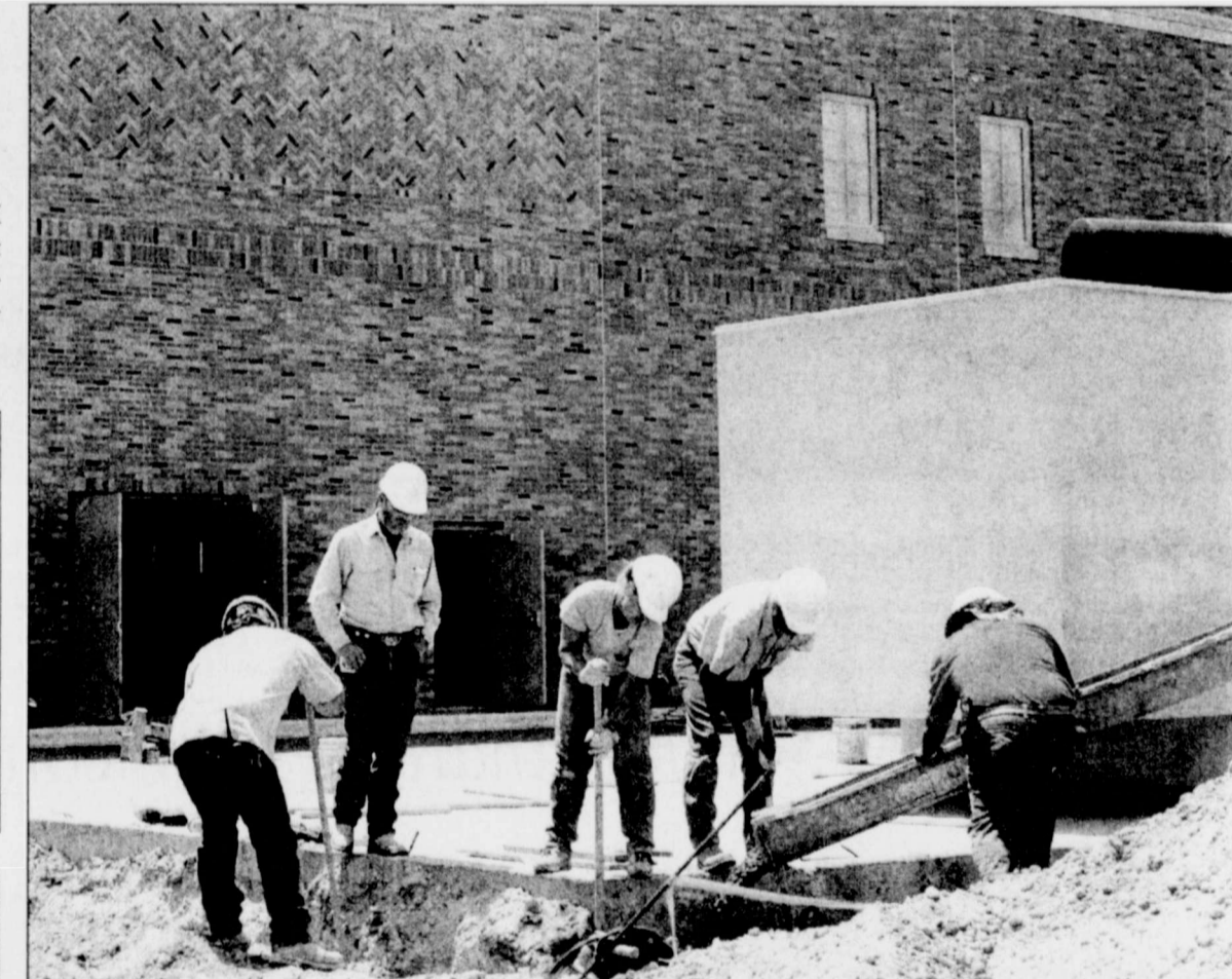
CONSTRUCTION WORKERS LAY the foundation for part of the new Animal Science building, which should be completed in October.
