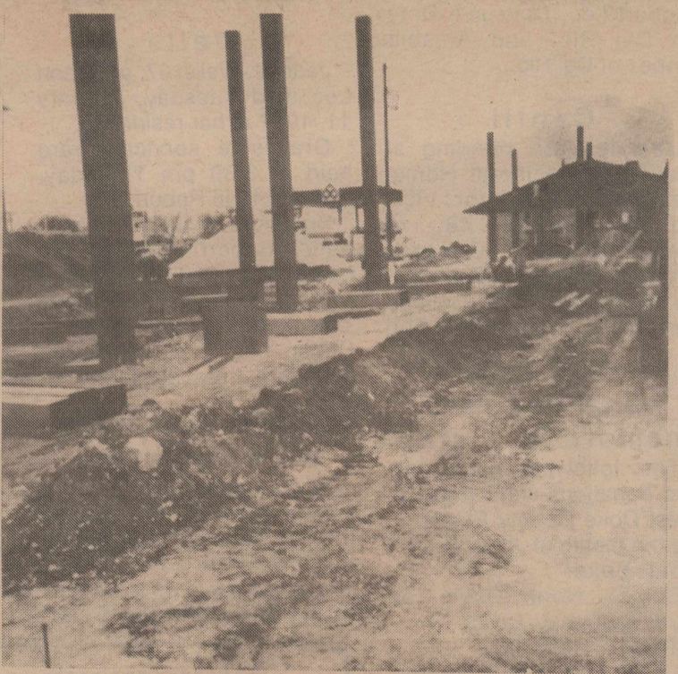
Work on the new Town & Country in Bronte is well underway. Crews are shown preparing the site for the gas and diesel tanks.
