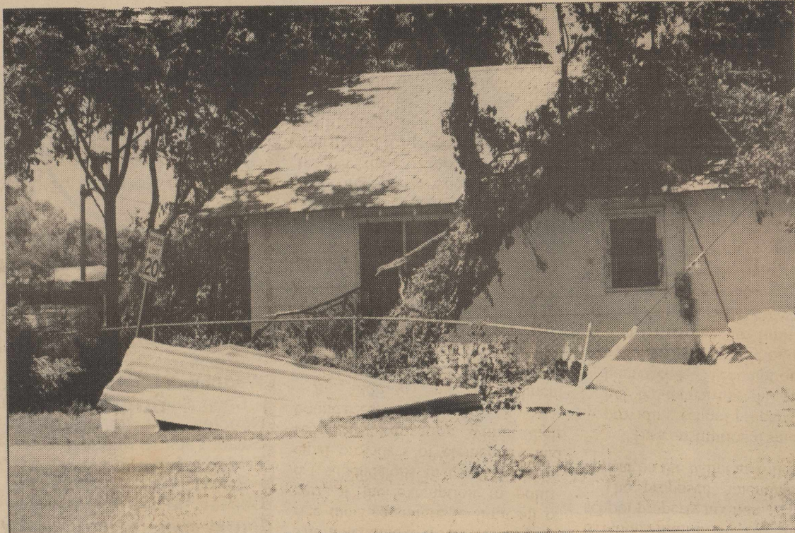
This house, belonging to Therell Burwick, was damaged during Thursday's Blackwell storm. The tin in the foreground is from the roof of the Church of Christ church across the street. Also, notice the large tree that went through the roof.
