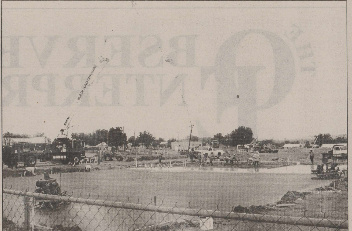
Lots and lots of concrete! W. B. Kibler Construction employees pour the concrete for part of the wing of the new Robert Lee High School facility. According to Superintendent Aaron Hood, some of the structure of the high school is expected to be standing by mid-July. As to all the other digging and holes throughout the construction site, Hood explains that most of the excavation is for drainage purposes. He also explained that they are working on the front parking lot, which should be ready by the beginning of the school year.
