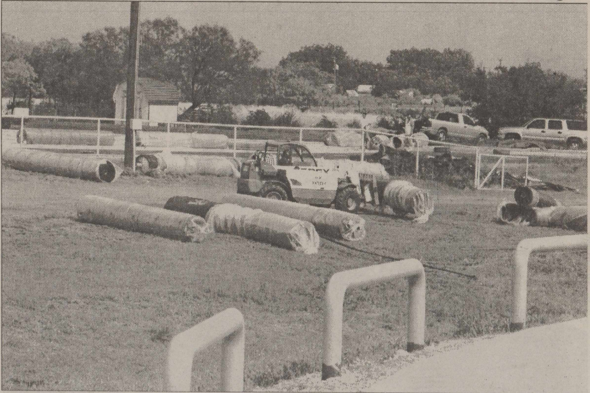
New Bronte Football Stadium! Progress continues on the new football stadium in Bronte. Workers unload large rolls of artificial turf.
