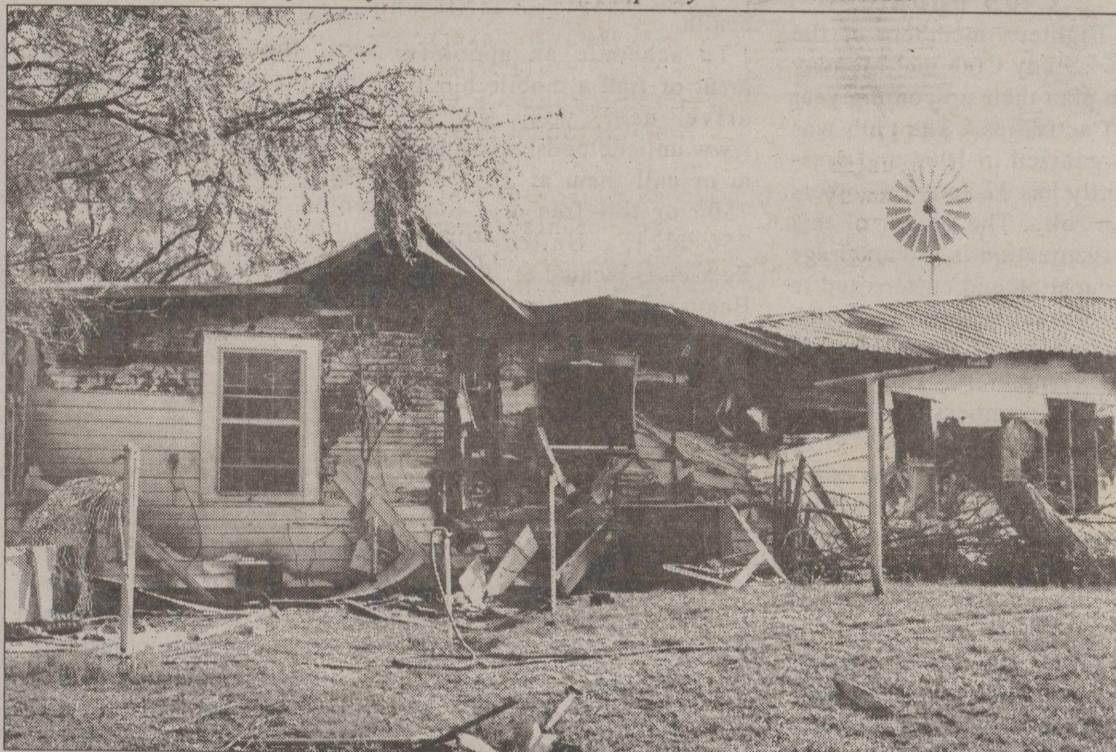
The donation is in memory of a recent house fire at the Caryl and Sonny Benton residence on Dripping Springs Road (shown below). The old ranch home was built in 1940 by the Carwiles. Despite the best efforts of local firemen, the home was pretty much a total loss.
