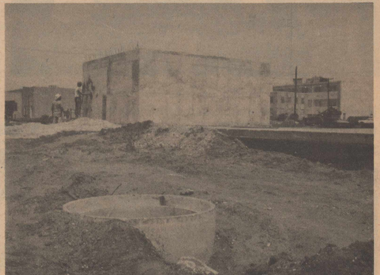
A progress report on the Seminole State Bank. A floor section and vault section are shown at the bank's new location at the southeast corner of the square. The courthouse can be seen on the right. In the foreground can be seen the entrance to the underground passageway to the drive-in tellers. (Not for people but for moneys and instruments to be sent back and forth.)
