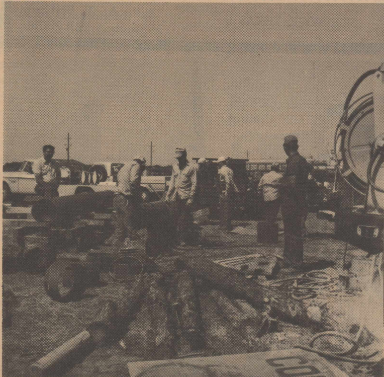
Great Plains Construction Company employees are shown at their office and yard on the Lamesa Highway. They are part of the 120-130 men who will build the 16' line from Denver City to McCamey, connecting the Shell plants.
