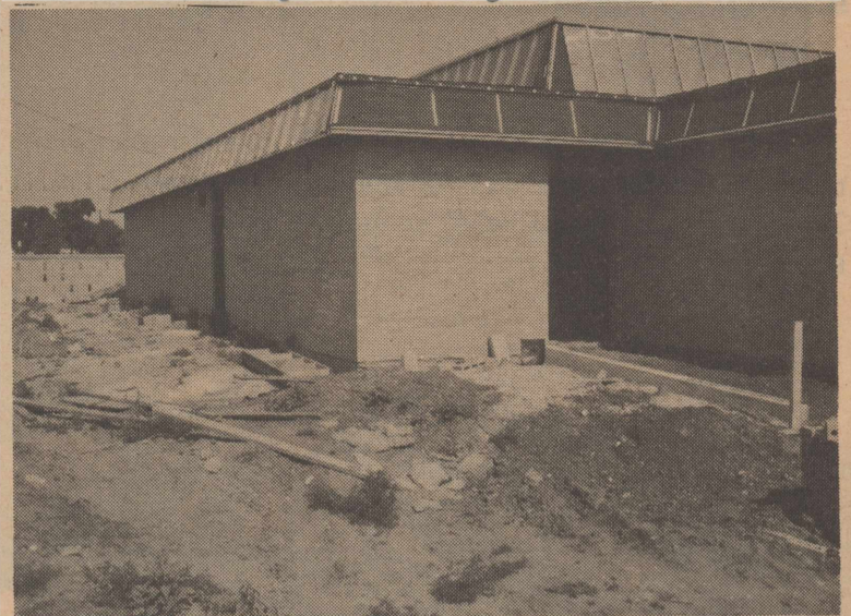
Construction on the M. S. Doss Scout Center is progressing daily. Note the new wall in the far background and especially the copper plating partially completed on the roof.
