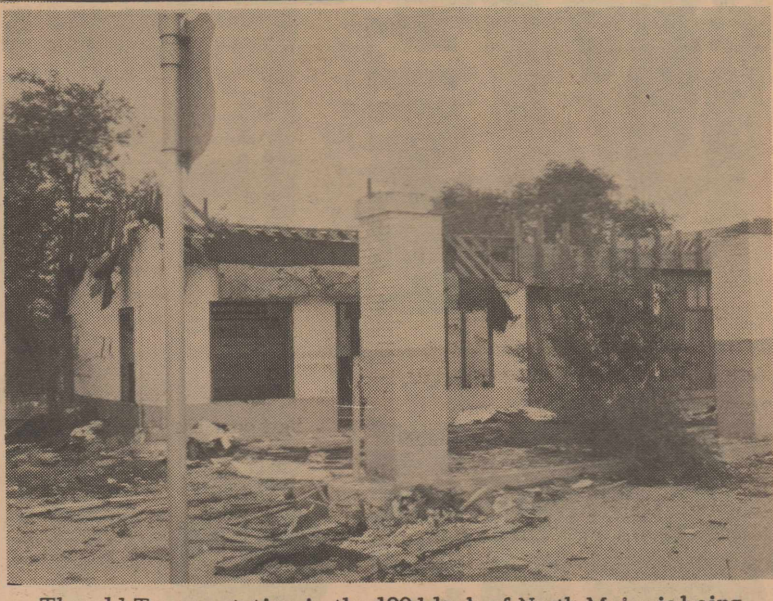
The old Texaco station in the 100 block of North Main is being torn down after serving the community 32 years. It was built by W. M. Adams, a Texaco bulk agent from Brownfield, in 1938. Ramsey Longbotham and Joe Anderson moved into it as its first operators. "When Ramsey (W.W. II war casualty from Gaines County) had to go to the service, I bought him out," said Joe. In 1944 G.B. Warneke bought the station from Andersons. Another operator was Bud Wilcox in 1952 and others. Mr. Pittman, who owns the Pittman Building next door, is having the building razed. One of the brick columns is rounded off on one corner where drivers have hit it.
