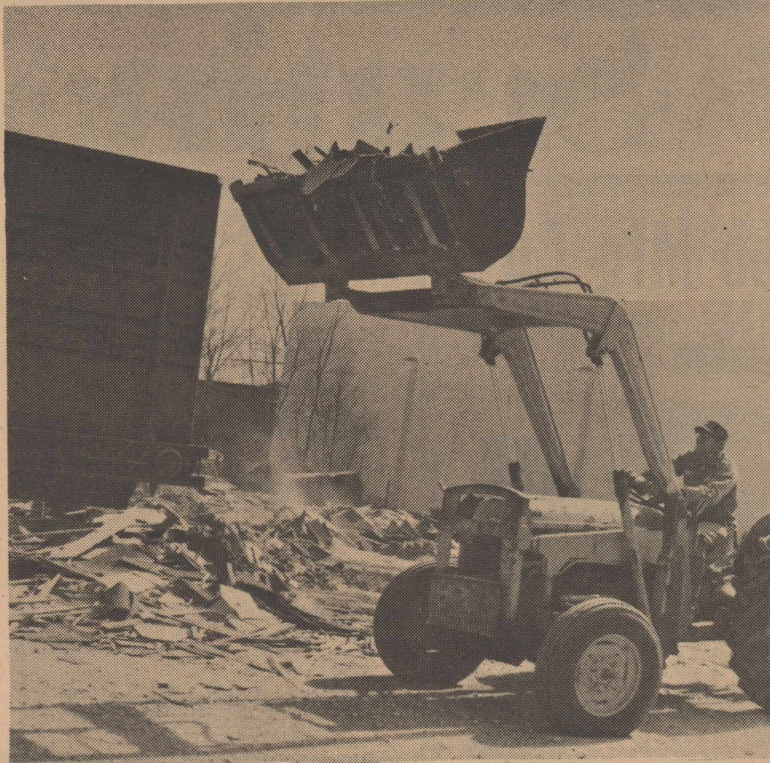
Another old dwelling is cleaned up and hauled off between Anderson & Sons Welding and TV Cable offices. Ray Anderson is cleaning up the last of the debris. Sixty-five to seventy-five old houses have been cleared out, others need to go.
