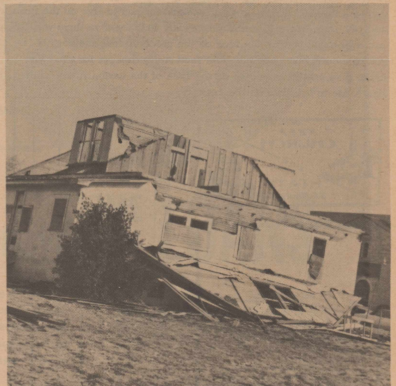
The Clean-up Campaign continues from last season. The old Eubanks house, across from the school, can be seen as it is being dismantled. The Clean-up Campaign is set for April 26- May 1 this year and will concentrate on the removal of old cars.
