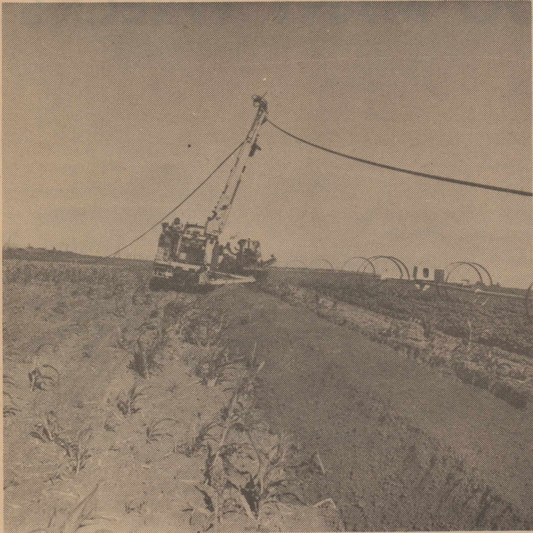
The underground cable of the telephone line is being moved west of Seminole. Note the side boom and the ditching machine as they are getting ready for the widening of U. S. Highway 62 west. An irrigation system can be seen adjacent to the work.
