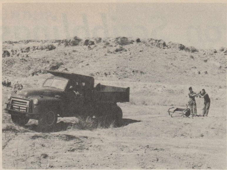
SMOOTHING down the wading pool beach at RAFB Buffalo Lakes resort are a group of men under the direction of Sgt. Charles R. McKinney of Personnel Services. Shown operating a grader are (l. to r.) PFC Henry Glasscock, truck driver, PFC Joseph Bruzzo and Sergeant McKinney.
