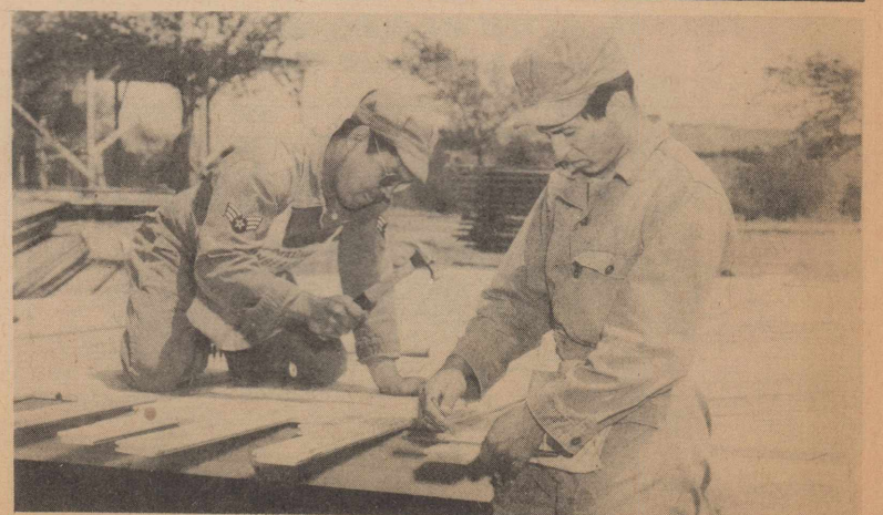
CARPENTERS CONSTRUCT PAVILLION — Air Installation carpenters from Reese Air Force Base are shown hard at work on a floor for one of the five pavilions presently being built on a picnic site at Buffalo Lakes. The carpenters are, left to right, Sgt. G. H. Dela Rosa and Pvt. Raymundo Gabaldon.
