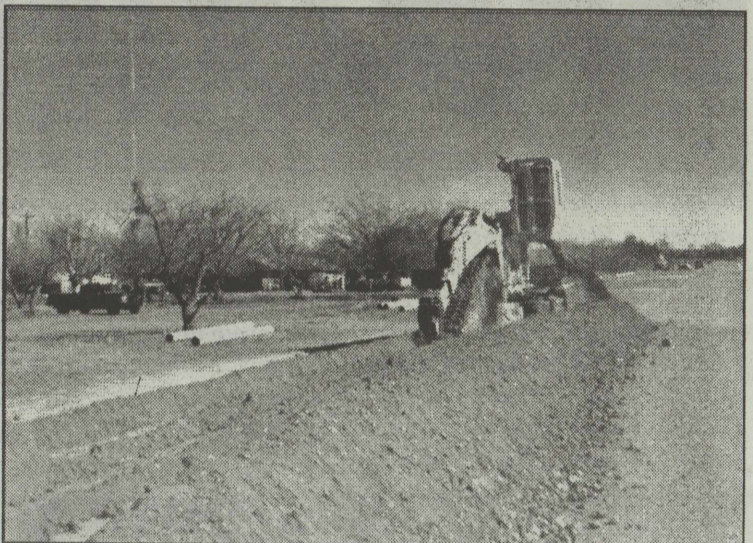
It's Begun! The construction of the trench for the water pipeline began Tuesday, January 17, 2012. The huge machine, along with the operator, were donated by Vermeer.
