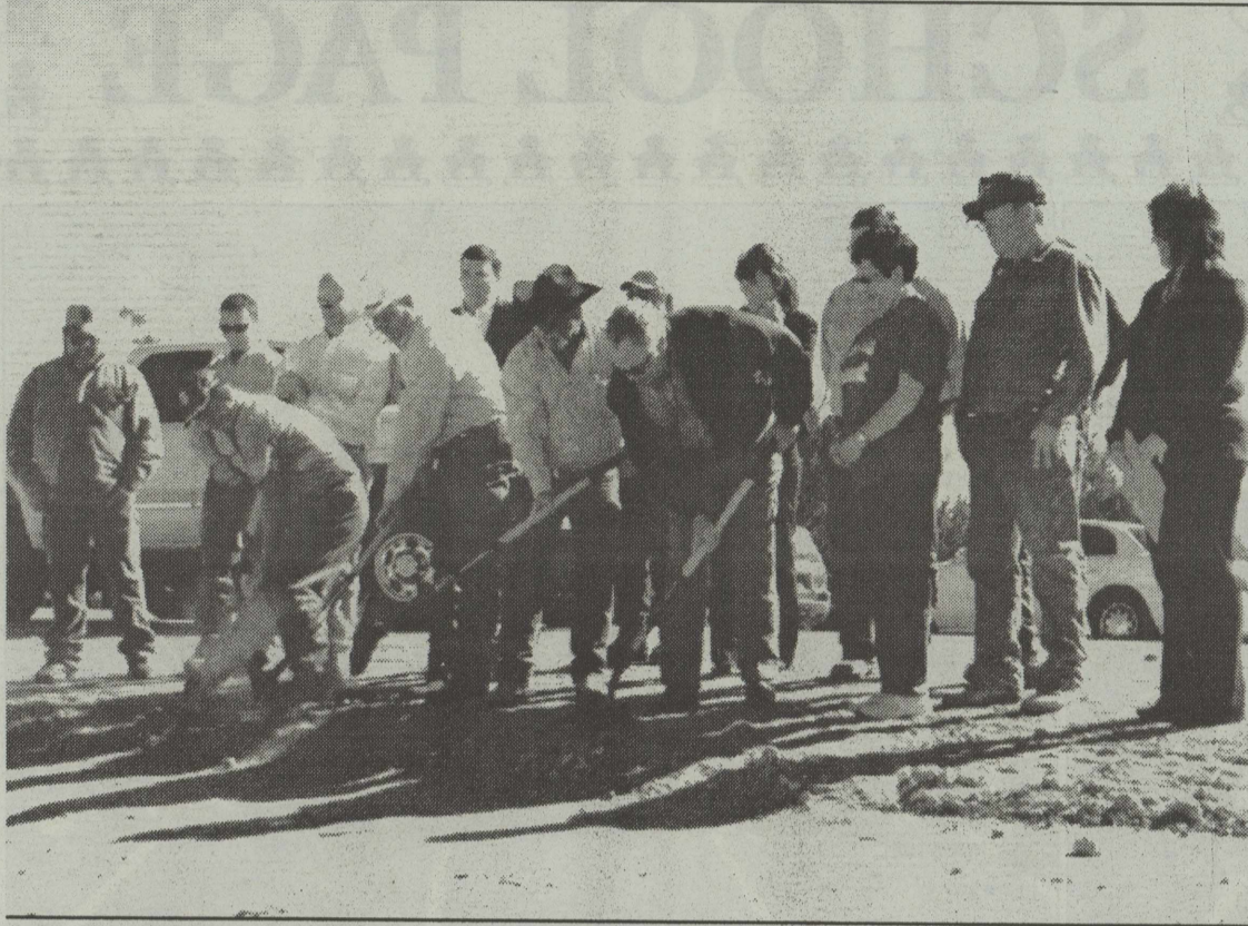
Pipeline Groundbreaking! Robert Lee City officials were joined by Coke County officials, State Representative Drew Darby, USDA representatives, Vermeer representatives, project engineers, and many others at the water pipeline groundbreaking ceremony held Friday, January 20, 2012.
