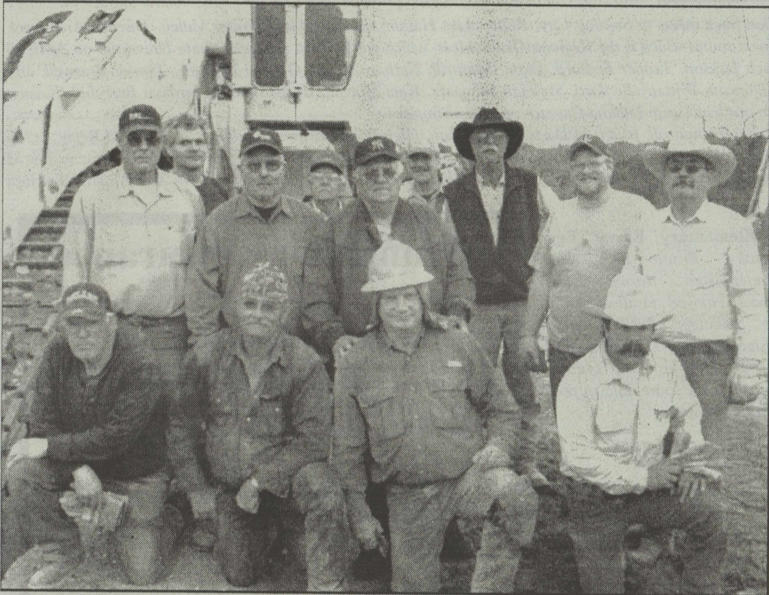
Pipeline Volunteers! This group of volunteers worked late on Thursday, February 2, 2012, to complete the 4.5 mile portion of the waterline to Bronte. The pipeline contractor was responsible for the remaining 7.5 miles to the treatment facility in Bronte.
