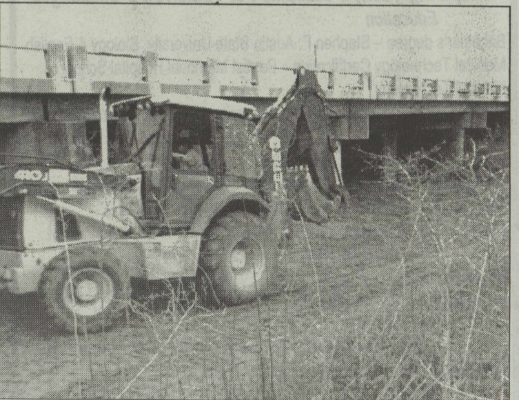
Water Pipeline! Roberts Construction of San Angelo began their section of the water pipeline at the Bronte water treatment plant. They are shown in late February 2012 covering up the section of pipe under the bridge over Highway 158 at the west edge of Bronte. Texas Water and Soil Company of San Angelo picked up where Robert Lee's volunteer requirement ended and headed west. They continued west to Double Barrel Road and then turned north to meet the Roberts Construction section at the intersection of Hwy 158 and Double Barrel Road.
