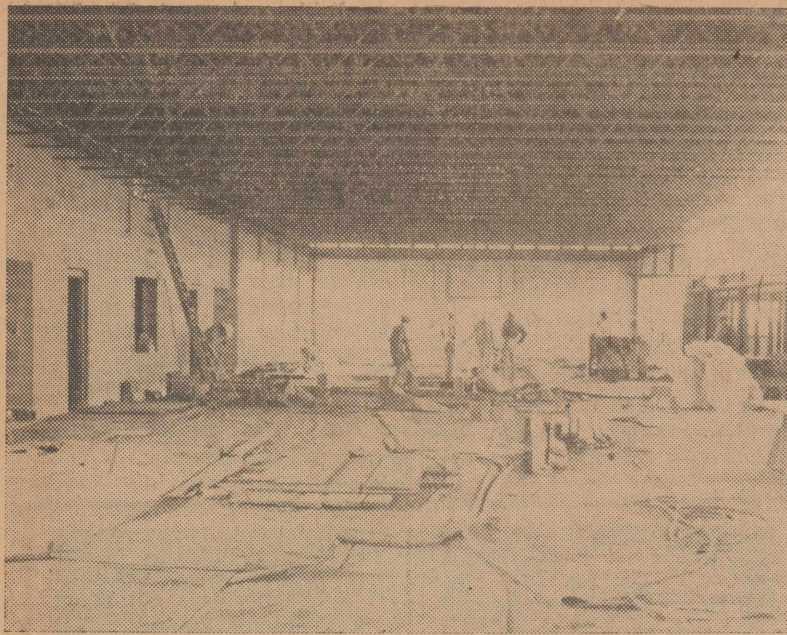
NEW MESS HALL —Construction workers complete preparations before pouring in the dining hall floor at one of the three building projects on the base. Plans call for the dining hall, and two dormitories to be completed in December. (Photo By Rushing)
