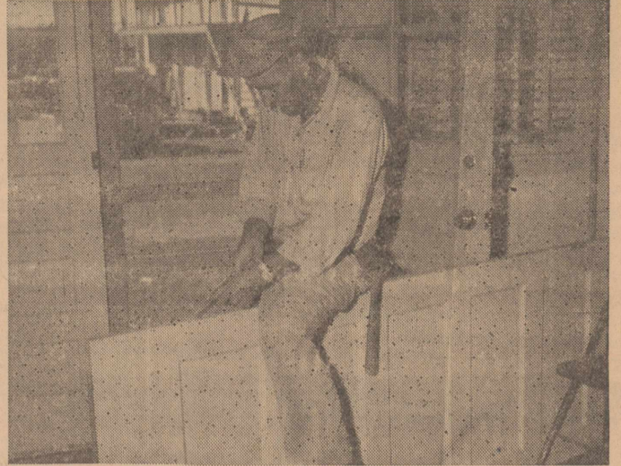
IT WILL SWING BETTER —William C. Cowan, at Reese since 1949, prepares the area for a new hinge which will lift a sagging door in the legal office. It's part of the Preventive Maintenance work he has been doing for 14 years on military installations, plus 3 years in service.
