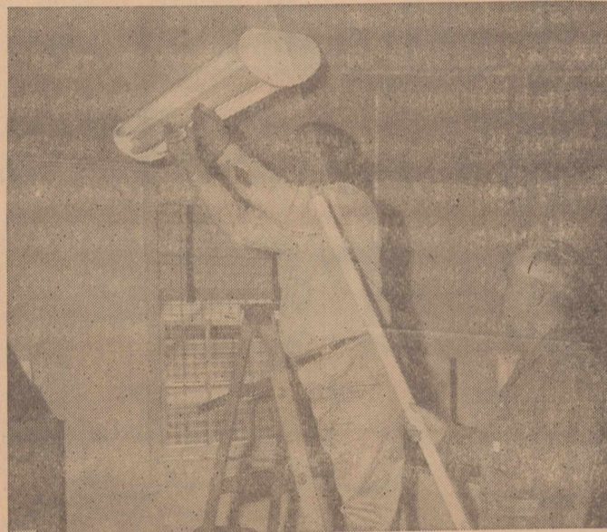
FOR BETTER LIGHT —Electricians make frequent rounds of buildings to check on lights, switches, and wiring. Here Bob Gregory installs a light, assisted by E. M. Gross.
