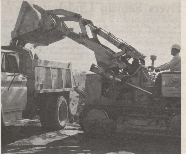
CONSTRUCTION —Workman of the C. M. Pharr Construction Company of Lubbock clear the ground as work started on the new gymnasium. The new gym is being constructed on what has been the tennis court.
