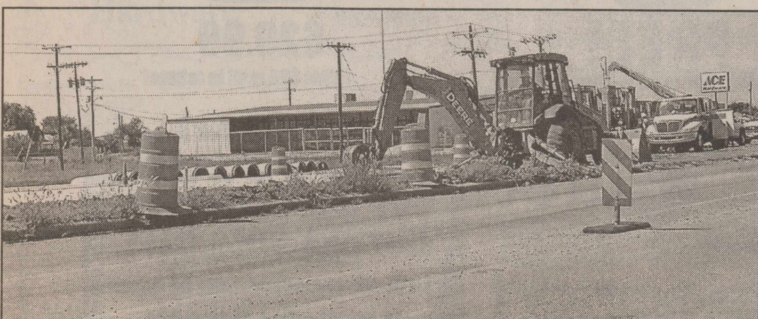
FLOYDADA "Y" CONSTRUCTION PROGRESSING--Dry weather is helping the "Y" construction and improvements continue. Crews have been very busy at the intersection.
