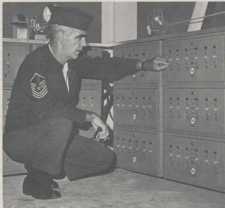
NEW ALARM SYSTEM—SMSgt. Charles H. Whittler, deputy fire chief, checks out the new fire alarm system in the base's new fire station (bldg. P-74). The system has a warning light on the master panel shown for each building on base which is tripped automatically in the event of a fire in that building. All of the facilities of the base's new fire station will be open for inspection by Reesites from 1 to 4 p.m. Monday through Oct. 8 as Reese observes Fire Prevention Week. (U. S. Air Force Photo)
