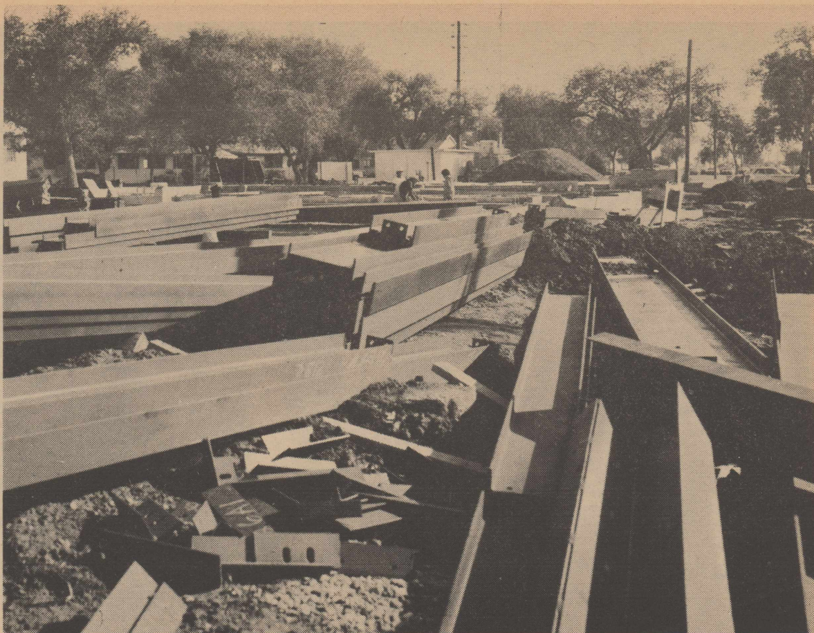
NEW THEATER —Construction on the new base theater seems to have picked up its pace recently as these steel beams have now been set in place. Located on base across from the bank, the new facility is expected to be completed by January of next year, according to Civil Engineering officials. (U.S. Air Force Photo)
