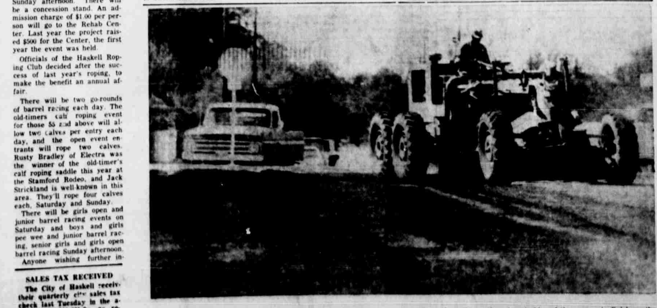
PAVING FINISHED AROUND THE SQUARE —The big machines moved in this week on the south and east sides of the square to finish up the job of cutting back the sidewalks and paving that began several weeks ago. (Photo by Don Comedy)
