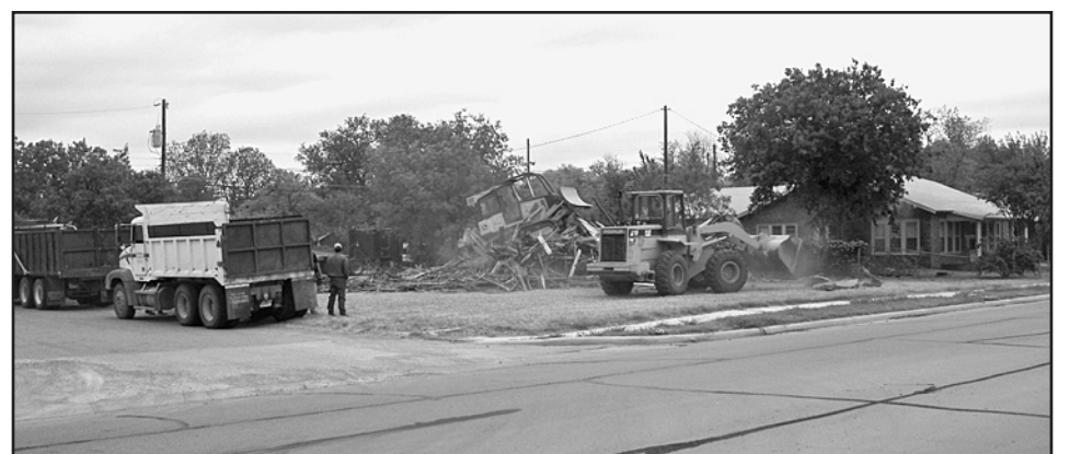
HOUSE DEMOLITION —City of Haskell and Haskell County work crews demolished several houses in Haskell last week to help with the beautification efforts. This house stood at the corner of N. 5th and Avenue E.
