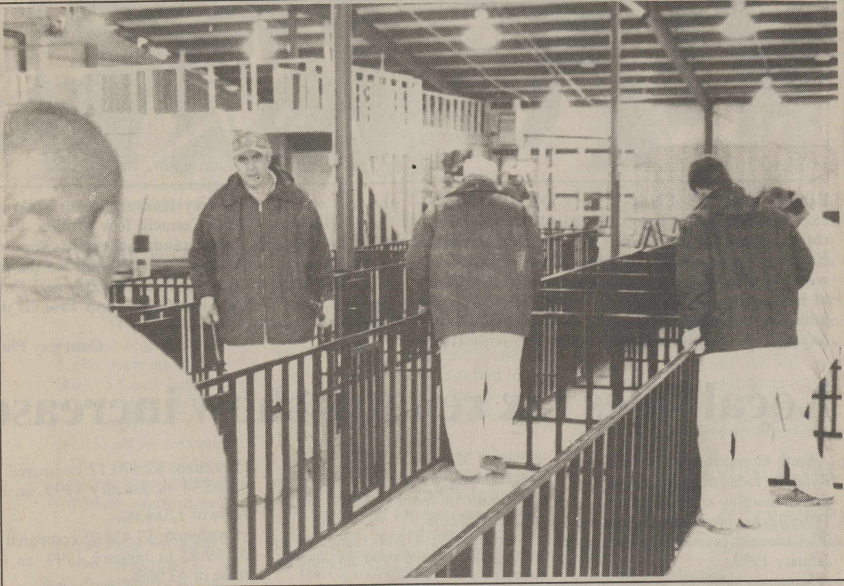
SHOW BARN CONVERSION-- Trustees from the Marshall Formby Unit of Plainview are continuing to assist contractors at the Unity Center with final preparations for the Center's first event--the Floyd County Livestock Show this weekend. The trustees are busy here erecting portable holding pens for animals.
