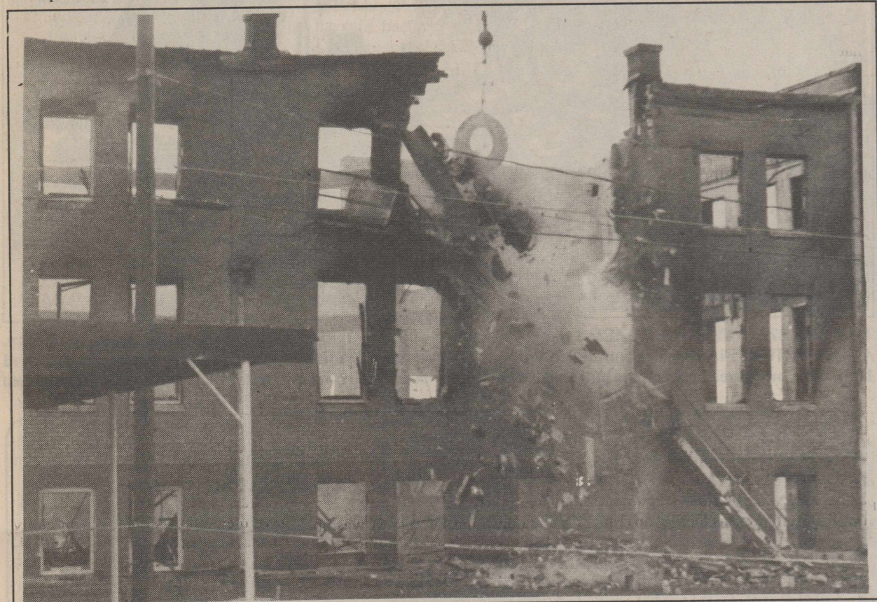
COMING DOWN -The wrecking ball is shown bringing down the dangerous walls of the fire ravaged Sunday School building of the First Baptist Church. Officials believe the fire started in the corner of the building in a utility room. (see related story) Staff Photo
