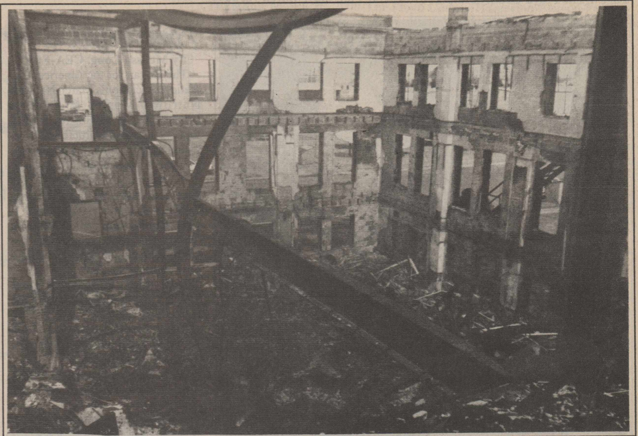
LOOKS LIKE A WAR ZONE -The burned out rubble of the Sunday School Building at the First Baptist Church resembles a war zone picture. Taken three floors up this photo shows the fire's destruction as the floors fell into the basement. (see related story) Staff Photo
