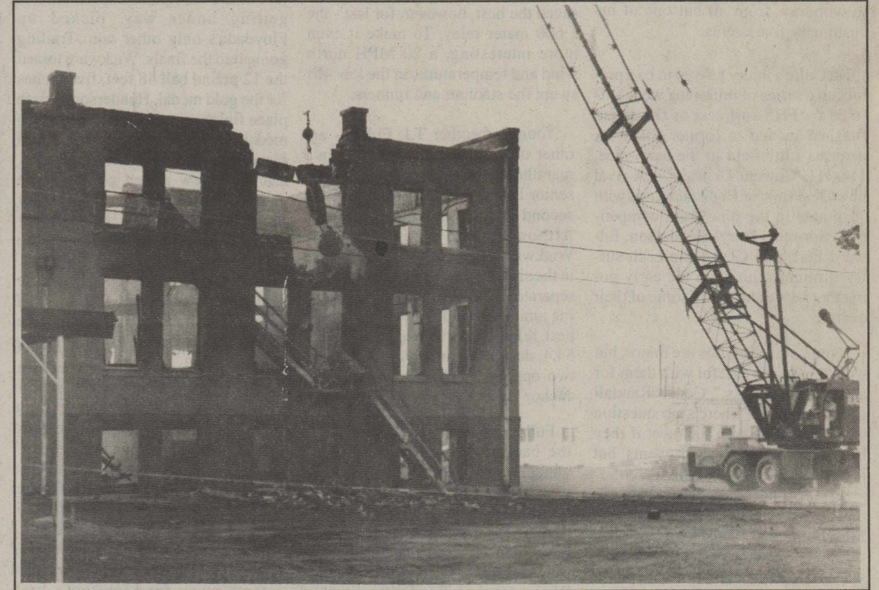
WHAT A DIFFERENCE A DAY MAKES -The day after the First Baptist Church's fire, which gutted the old auditorium and the Sunday School building, demolition crews were tearing down the dangerous brick walls. The fire brought in fire fighters from all the surrounding towns to help control the blaze. Staff Photo
