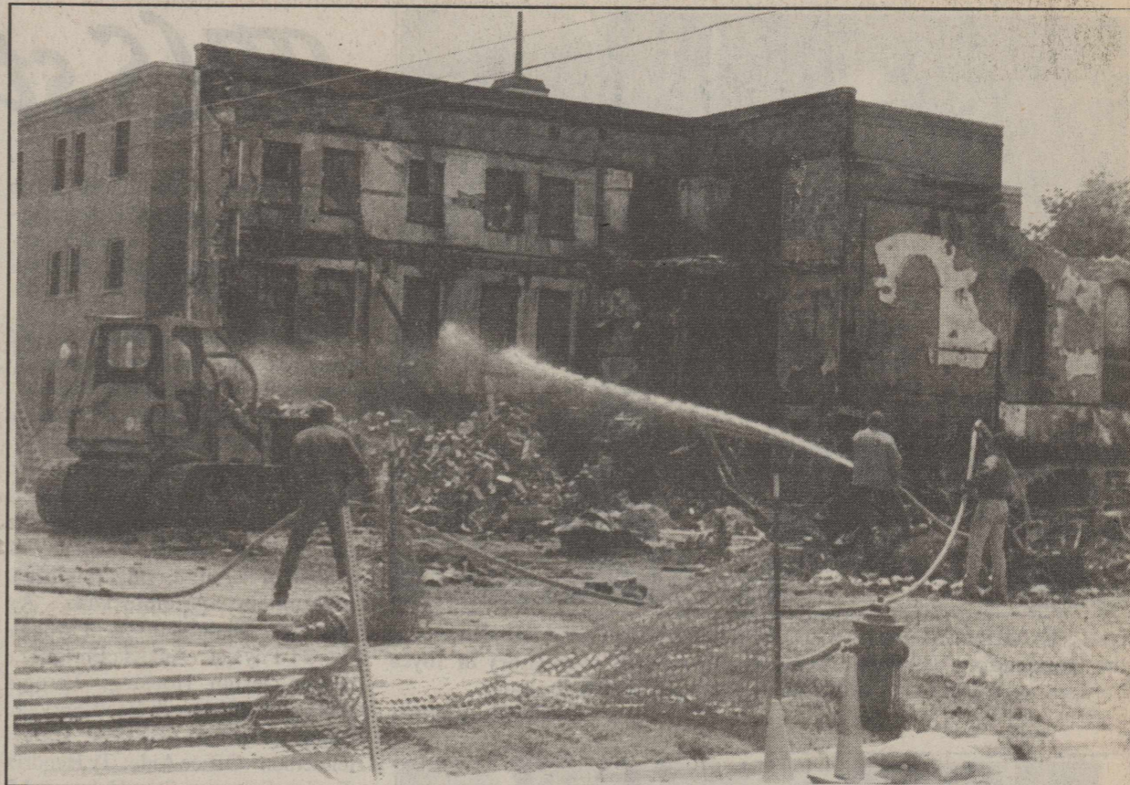
FLOYDADA. The fire destroyed both the old sanctuary and rubble were being removed this week from the remains of the March 12th fire at the First Baptist Church in Floydada. The fire destroyed both the old sanctuary, the Sunday school building, and severely damaged the church offices. Staff Photo
