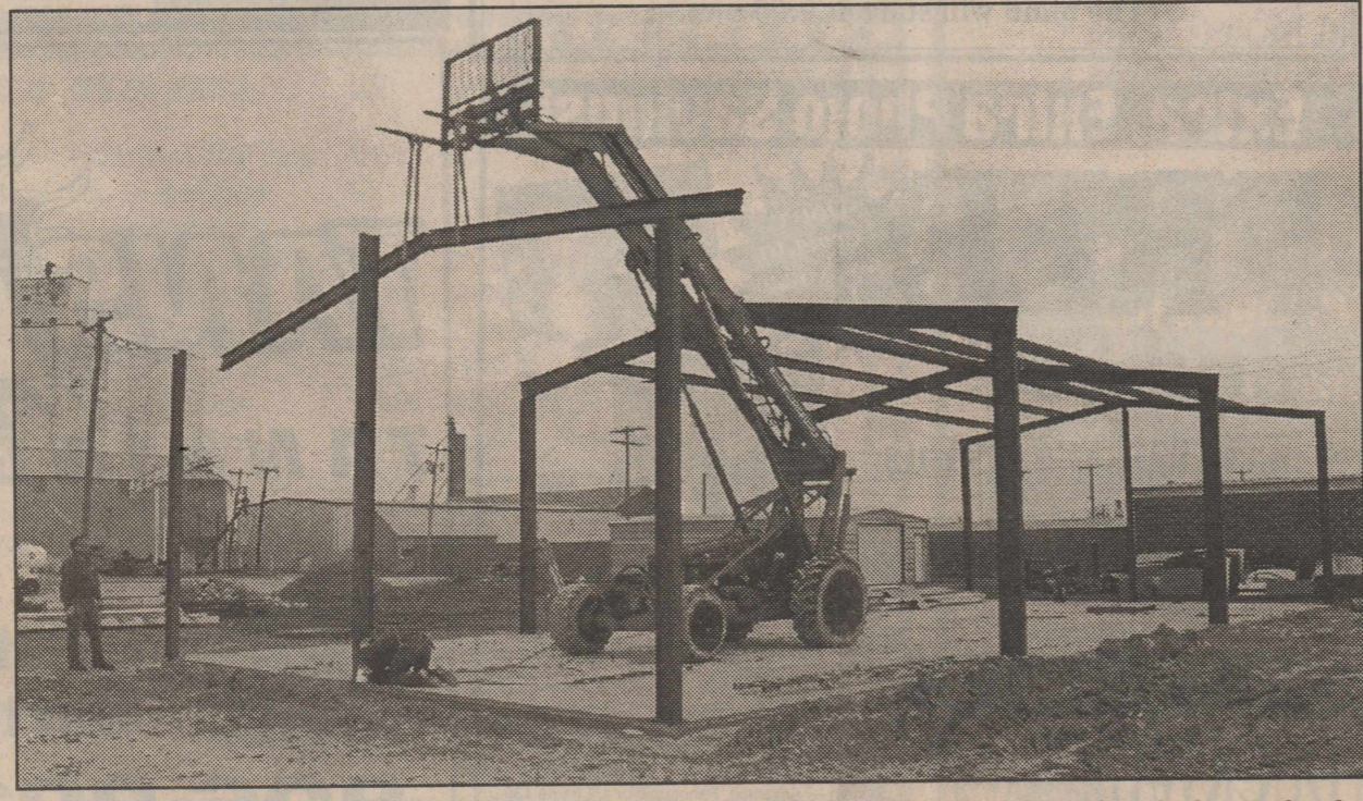
VOCATIONAL INSTRUCTIONAL BUILDING GOES UP --Ed Marks Construction raises the beams for the PAC's Vocational Instructional Program (V.I.P.) building across the street from PAC in Floydada. The building will be used to teach PAC youth the skills of general automotive repair. Staff Photo
