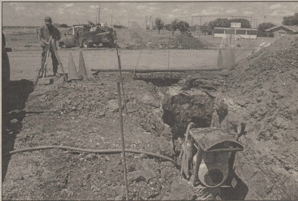
CLEARING THE WAY--Kelly Williamson and Richard Tuz bore under FM #2301 to clear the way for the Aiken to Lockney water pipeline. Staff Photo
