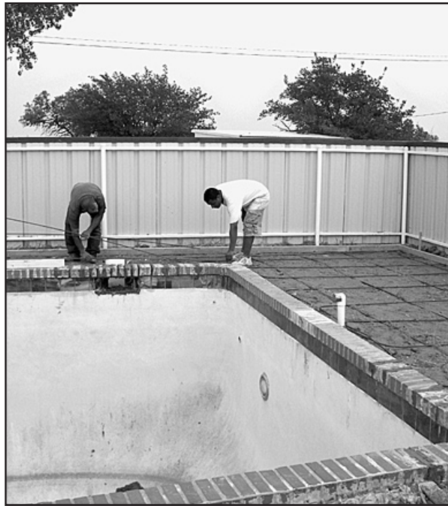
POOL REPAIRS —The swimming pool at the Haskell Country Club is receiving new tiles around the top of the pool and a new surface around the pool. Paul Rodriguez, left, and Tony DeLorosa are preparing the reinforcing steel before the pouring of the surface. The men are from Lubbock.
