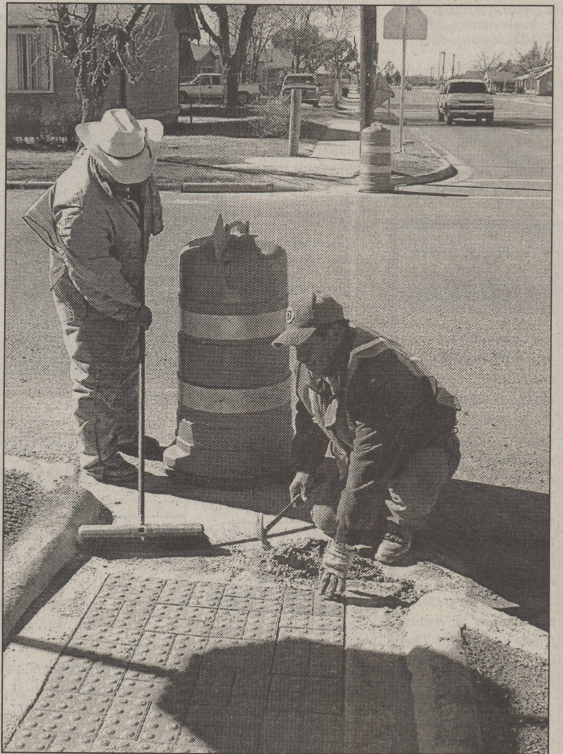
WHEELCHAIR RAMPS GOING INTO PLACE-(l-r) Tavarez Manuel and Manuel Rodriguez of Odessa are shown Tuesday afternoon laying the brickwork for State and Federal mandated wheelchair ramps being placed at the intersections on Houston Street in Floydada. Staff Photo
