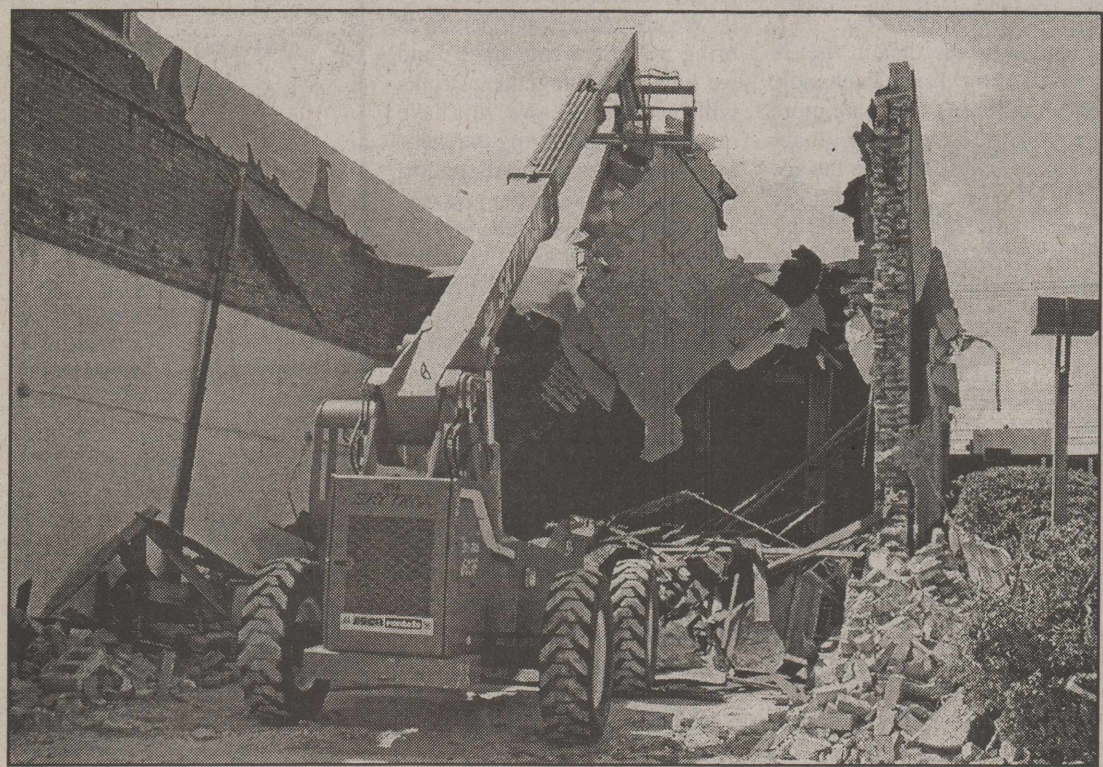
REMODELING AT FNB OF FLOYDADA --Workmen are shown tearing down the north wing of the First National Bank of Floydada Tuesday. The rubble is being hauled away by dump trucks. FNB President Tom Farris told the Hesperian-Beacon, "We are moving the drive-in window back into the main building and expanding our drive-in lanes. Work should be finished by this fall. Staff Photo
