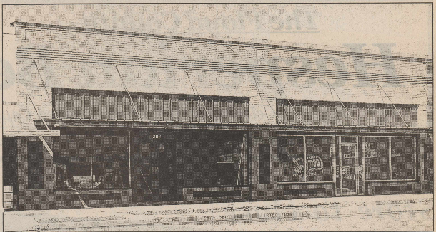
MCDONALD CONSTRUCTION TAKES ON NEW LOOK--In an effort to help the City of Lockney in their Downtown Beautification project, Marlon McDonald and Danny Bowman worked for two weeks on the store front of their McDonald Construction building on Main Street in Lockney. The overhang was rebuilt and the front of the building was repainted. Staff Photo
