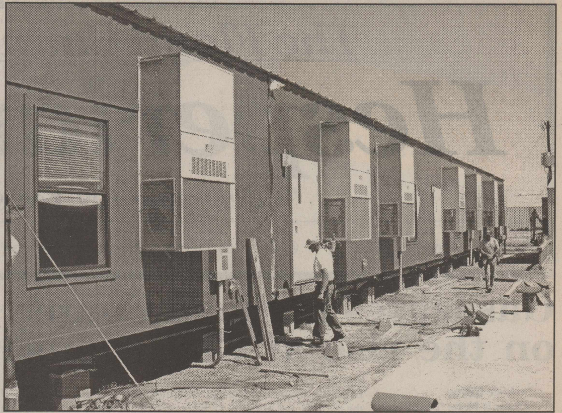
TEXAS MIGRANT COUNCIL'S NEW BUILDING GOING UP-Several portable buildings were seen Monday morning being installed together to make TMC's new facilities at the Floydada office. TMC Transportation/Facilities Coordinator Karen Poe of Lubbock told the Hesperian-Beacon, "This new building, which will be ready by June 30th, will take the place of the old facility. We plan on tearing down the old facility at a later date. That space will be used for parking and a playground. The new facility will have five new classrooms and four new offices. We already have two other module buildings that are two years old, which have two classrooms each. We are funded for 100 kids and 27 employees. We need more help right now and we are hiring. Our seasonal program is year around and our summer program is in progress now. We serve all migrant worker's kids here in Floydada from Lockney, to Ralls, and to Petersburg. Our other offices in this region are located in Plainview, Lubbock, Brownfield, Muleshoe and Hereford."
