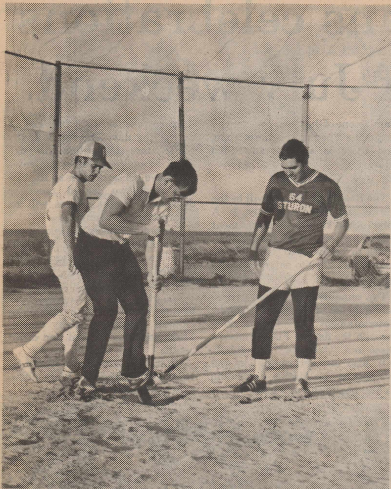
WORK, WORK, WORK — (Left to right) Bob Jones, Bill Davis and Cliff Napolitano dig out first base in preparation for sinking the bases in the ground during the repair and cleanup of the softball field. (U.S. Air Force photo by SSgt. Ron Pack)
