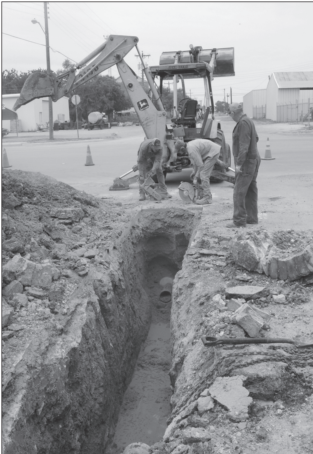
SEWER LINE IMPROVEMENTS—Tony Williams, far right, looks on as Kelly Williams, left, and Tyler Mitchell saw out the concrete along Hwy. 380 to allow them to finish digging to reach the existing sewer line connection seen just below where they are standing. The new sewer line at the bottom of the picture is a 12" line and replaces the old 6" line that runs south of the highway to the sewer plant on Avenue B East. The crew will cross the highway and head north for three blocks in the days to come replacing the line on the north side with a 10" line. The four block venture is a continuation of the bypass project and will bring improved sewer service to the prison complex.
