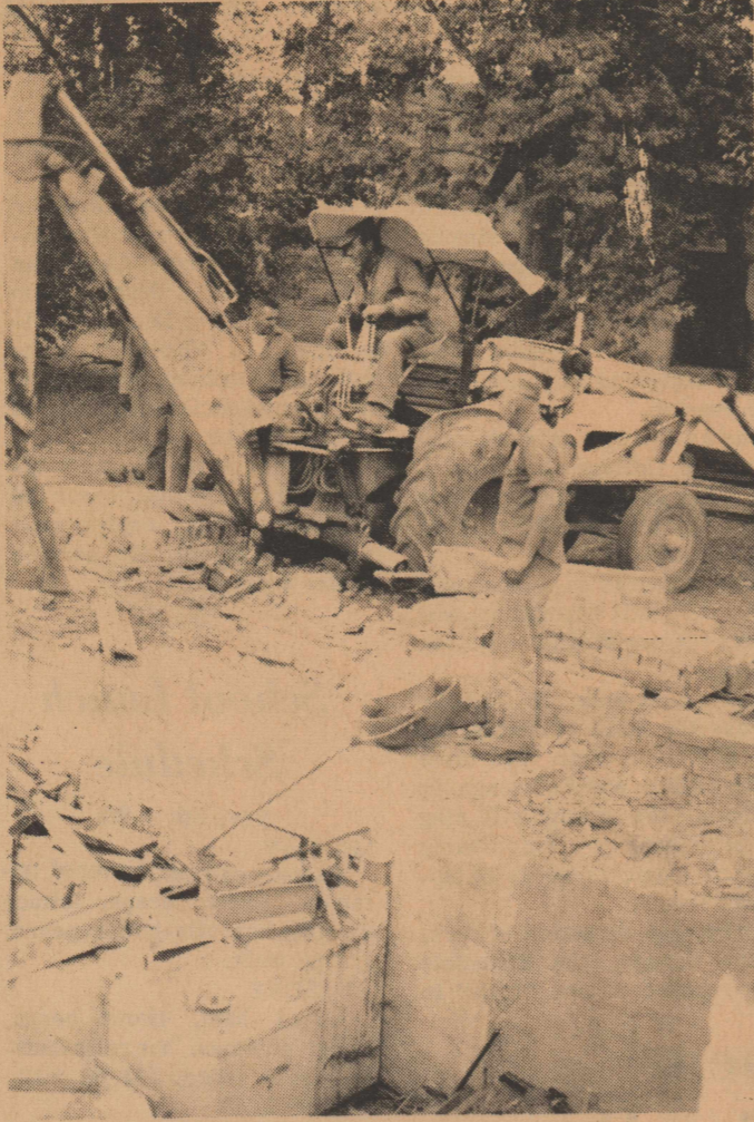
A LANDMARK TUMBLES DOWN --When this photo was taken we thought this old landmark was to be razed and filled in, the basement of the old Christian Church building, but it is still there. Shown above are workmen getting part of the debris out of the basement prior to the filling operation.
