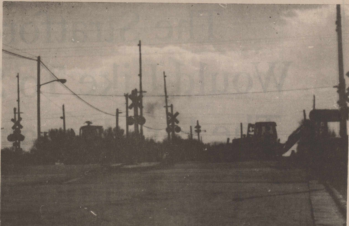
Construction has been under way since last Monday on the railroad crossing on Main Street. This should be finished soon.
