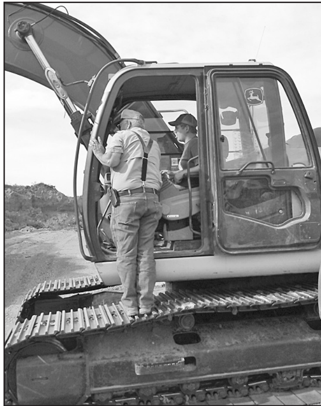
EXCAVATOR LESSON —Rochester Vo-Tech student Thomas Baker learns how to operate an excavator with tips from Bill Hester.
