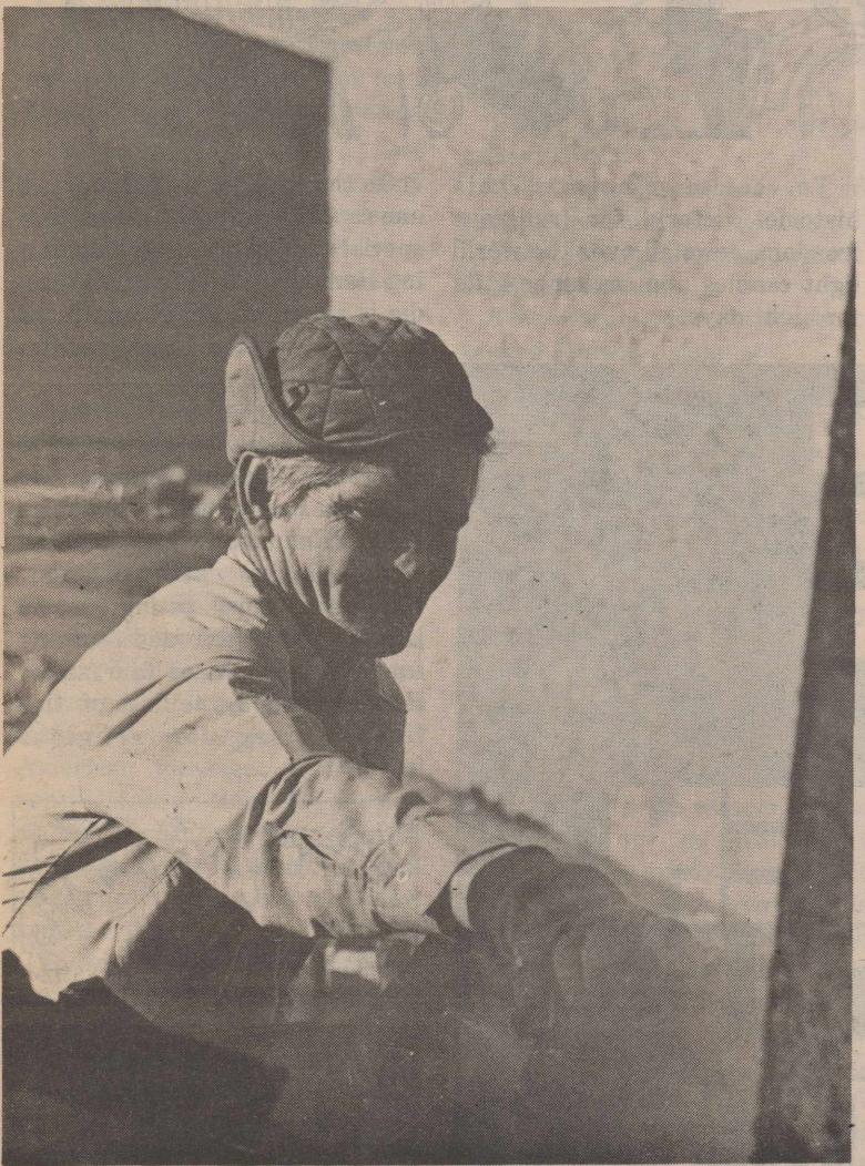
David Jones, top, cleans out the well for the transformer pad that will serve the new commissary. A 95-day delay brought about by changes in construction plans, government delays and weather difficulties will push the opening date back to late April. This will line up with the expected grand opening of the new Exchange facility. Gene Gartman feeds tar into the furnace to finish the roof of the building. (U.S. Air Force Photos)
