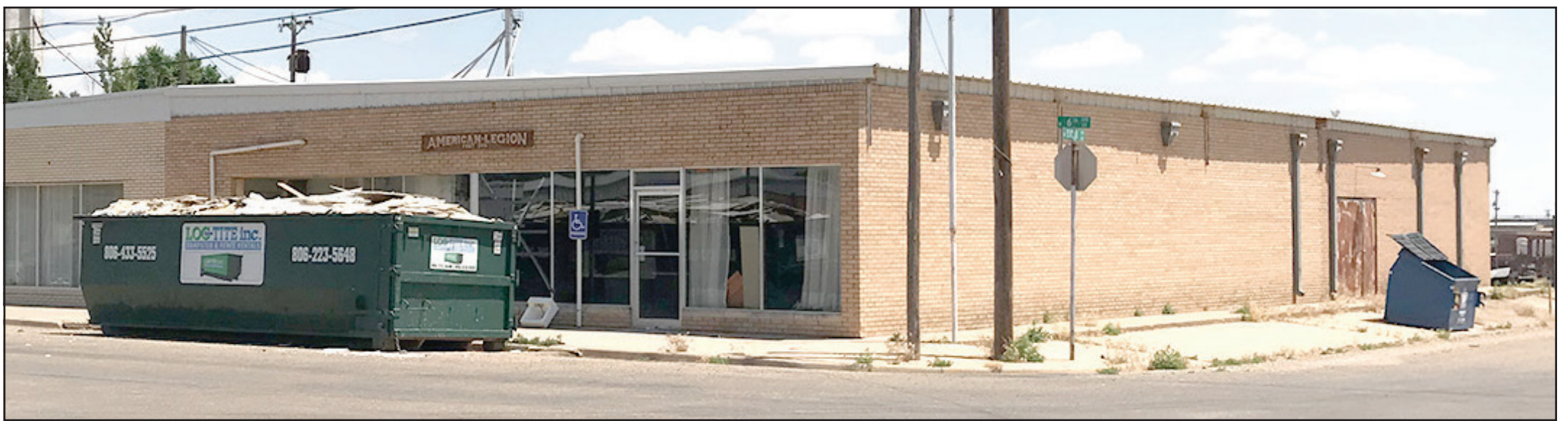
Work has begun on renovations at the American Legion building. The building was decided to the Parmer County Pioneer Heritage Museum and plans are to use the extra space for more exhibits. A large military exhibit showcasing Parmer County veterans is in the planning stages. The current ceiling is being removed and spray foam insulation will be applied. The roof will then be repaired. If you would like help with the project to restore the American Legion building, please send your donation to Parmer County Pioneer Heritage Museum, %Bruce Fleming, 1205 W. 9th Place, Friona, Texas 79035.
