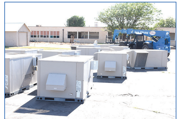
Workers removed the HVAC units from the Primary School building this week. Asbestos materials are also being removed as required by law. Demolition is currently scheduled to begin just after the July 4th holiday.
