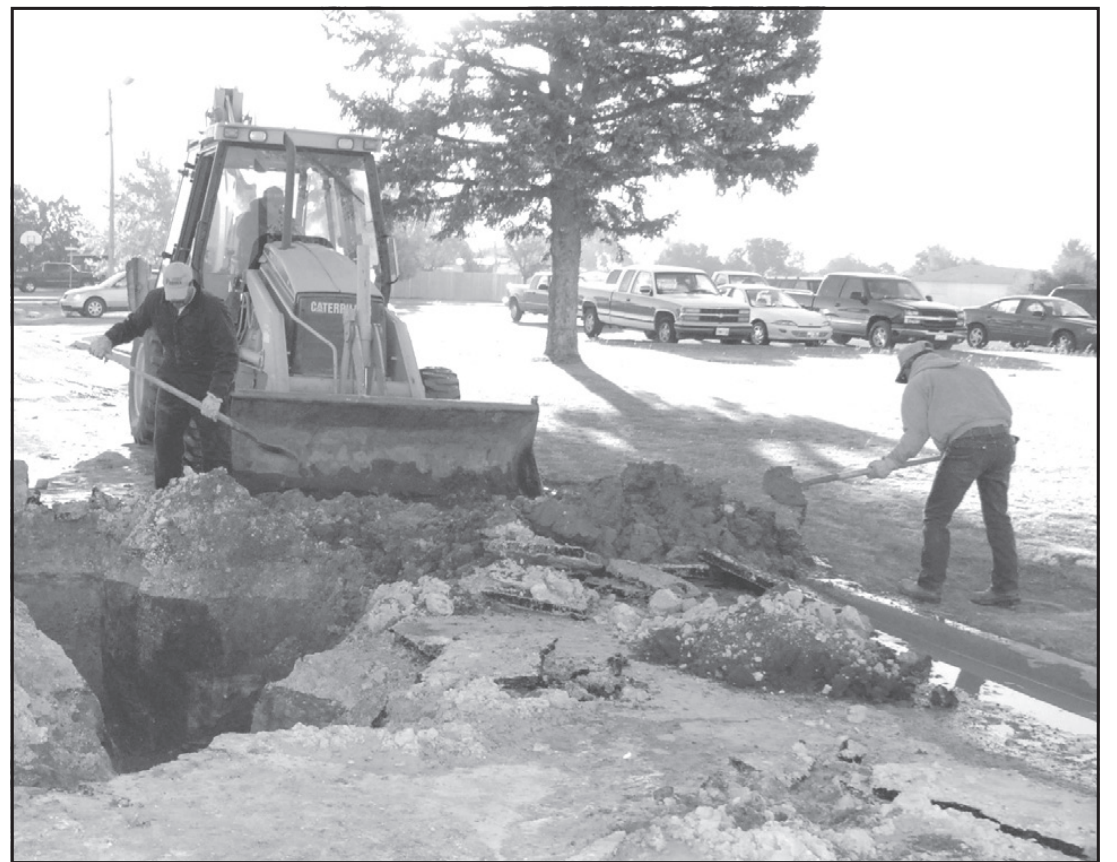
Friona city employees Richie Perez and Ted Osborn work to repair 14th Street after a major water main break late Monday kept the city crew busy until 1 a.m. Tuesday morning. The major water pipe served Parmer County Hospital and flooded the street before workers found the break and repaired it. The street was closed to traffic from Cleveland to White. Friona reported a low of 27.5 degrees overnight Monday but officials do not believe freezing caused the break. Ron Carr photo. (Friona Star, Thursday, October 25, 2007)
