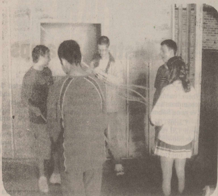
Shown at left: Cisco Networking Academy Students of Instructor Dan Hembree, wire the Imagination Station to set up the local and area network for the coming computer room to be open to the public. L/R: Josh Williams, Bill Walker, Carson Buckles, Heather Seiler, and Brian Kimbrough.
