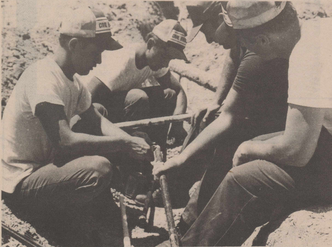
Members of the Sheppard team team up to put in new gas and water lines near the Reese sewage area.
