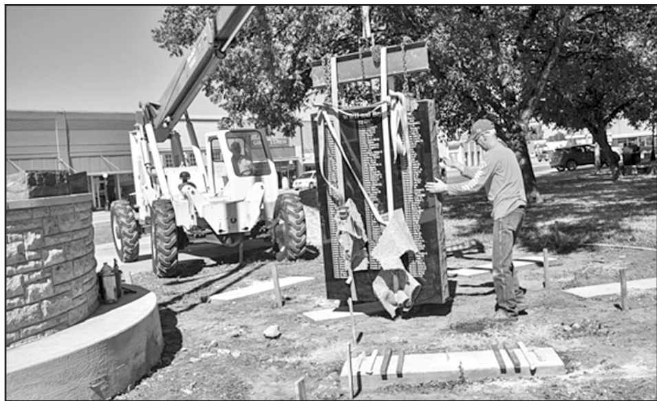
PROJECT STARTED —Three of the tablets for the Haskell County Veterans' Memorial were set this week. County Judge David Davis, running the crane, assisted the contractor Davey Vestal. The 10 tablets will be set in installments. Any names left off will be added to the last tablet.
