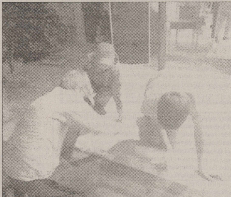
Laying the soundproofing and the wood laminate-AJ Riffe, Bret Barnard, and Russell Spurlock
