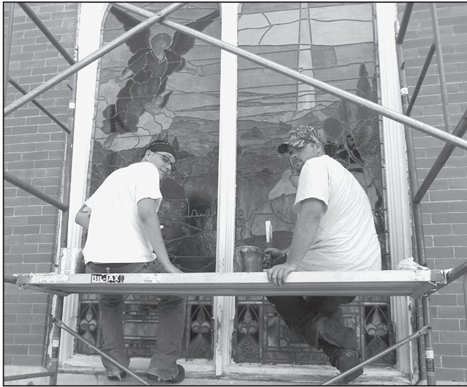
PROTECTS STAINED GLASS —Jason Eide, left, and Dustin Jonsgaard, right, are working on the stained glass restoration project underway at the First United Methodist Church in Haskell. They are restoring the lead in the windows, cleaning the glass, applying caulking, painting and finally, will cover the windows with a lexan covering that features a vented system to help preserve the windows for many years to come.
