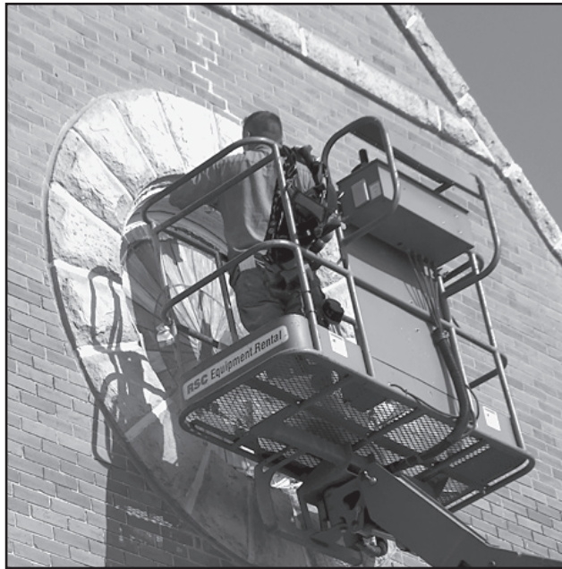
RESTORATION IN PROGRESS —Gaylin Eide of Willet Hauser Architectural Glass is shown atop the manlift preparing the circular stained glass window at the front of the First Methodist Church in Haskell for the restoration process. The company has been in business for over 100 years and works with churches and other institutions to design, repair, restore and protect their existing stained glass treasures.
