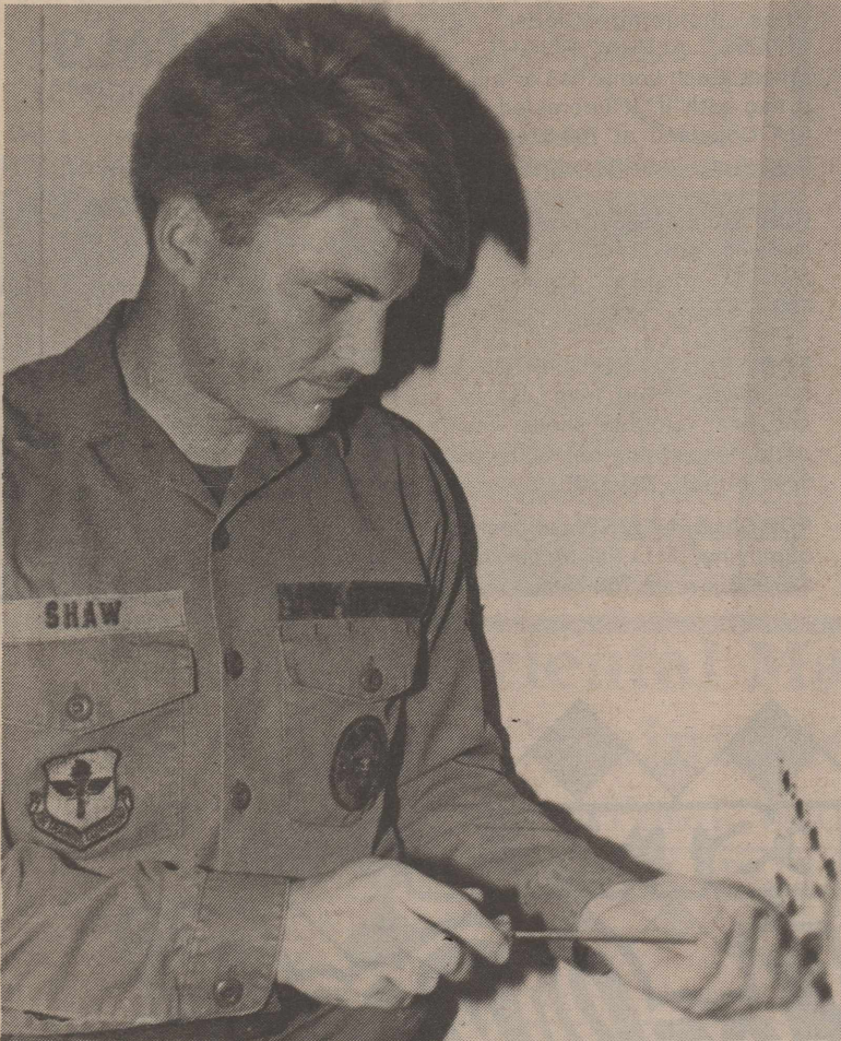
Amn. Ray Shaw, a 64th Civil Engineering Squadron electrician, replaces electrical outlets in the new Physical Fitness Center Annex. The new annex, a remodeled room of the Old Talon Inn next to the Mathis Recreation Center, will be used for aerobic exercise, martial arts and gymnastics.
