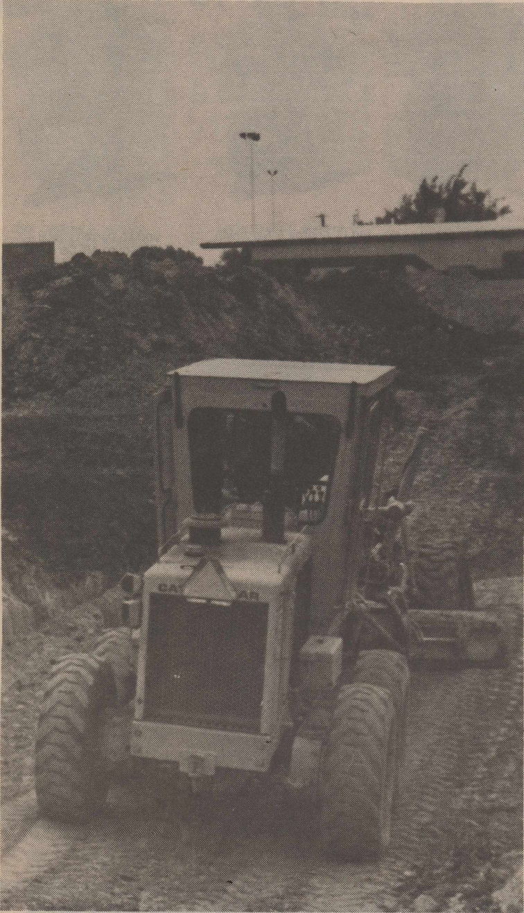
The second phase of the 64th Civil Engineering Squadron project is underway with the renovation of the Civil Engineering parking lot. The work is scheduled to be completed by the end of September. (USAF Photo)
